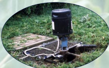
Effluent pumped to irrigator
